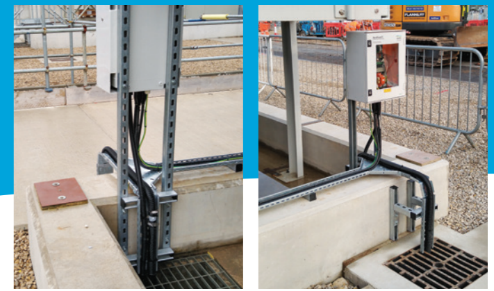
Bespoke special-build installation using National Grid specification enclosures, designed to interface with existing glycol alarm system.
